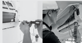
Difficult electrical connection
