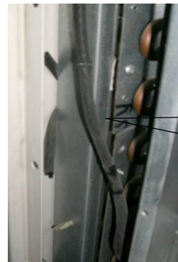
After being reconnected, the system becomes normal
